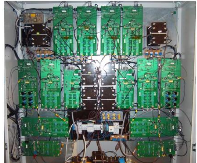
Medium Voltage 1-ph Cascaded Multilevel Converter (System 3)
